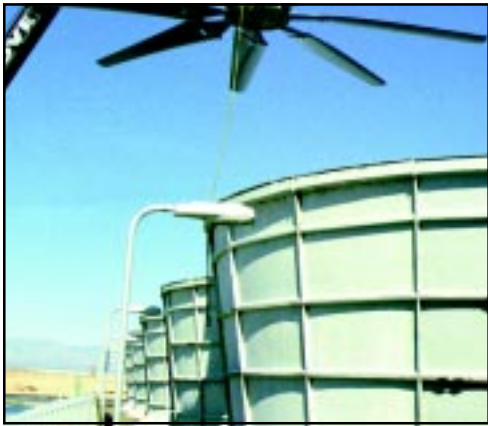
Typical Large Cooling Tower Fan with VR Stack Fig. 9
